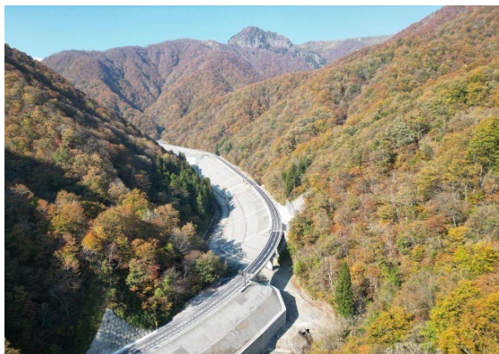
Improvement and pavement construction work at Kammuriyama Toge Road in Tsuka district (Kinki Regional Development Bureau, MLIT)
