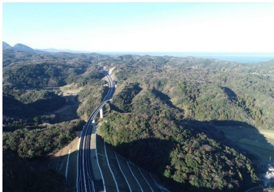
FY2022 Shizuma Nima Road pavement construction work in Isotake district (Chugoku Regional Development Bureau, MLIT)
